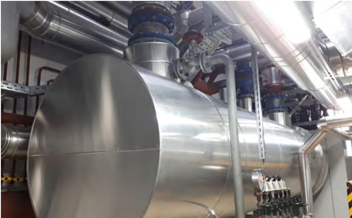
Power to Heat Anlage Thondorf
